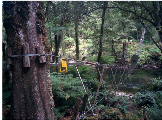
A bridge with low capacity
